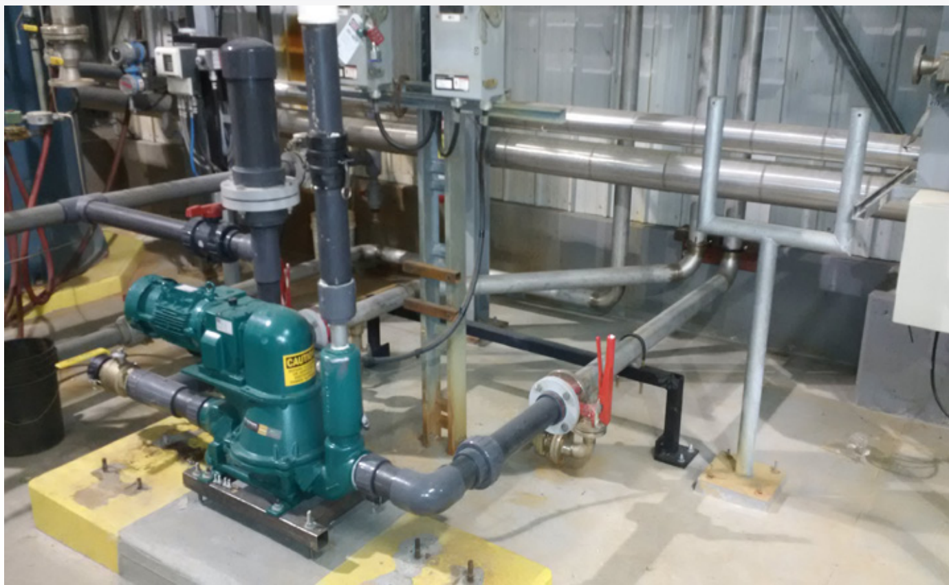
Mud Sucker 3FA-EC with a 3 hp Honda engine with up to 80 GPM fluid handling capabilities*. Shown on a military base pumping waste oil. Non-collapsible suction and discharge hoses are available.
