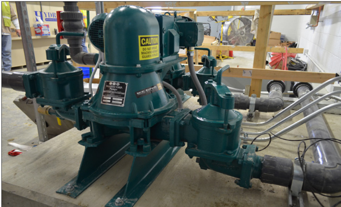
Mud Sucker B Series at a food processing facility. This application involves separating oil and waste water and then pumping for further treatment.
